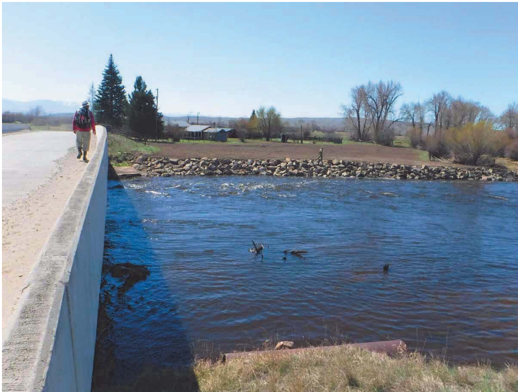
Figure 4. Right bank of Sub-Reach 5 in April 2016, following placement of bank stabilization (riprap). View is from upstream rail of Pennington Bridge.
