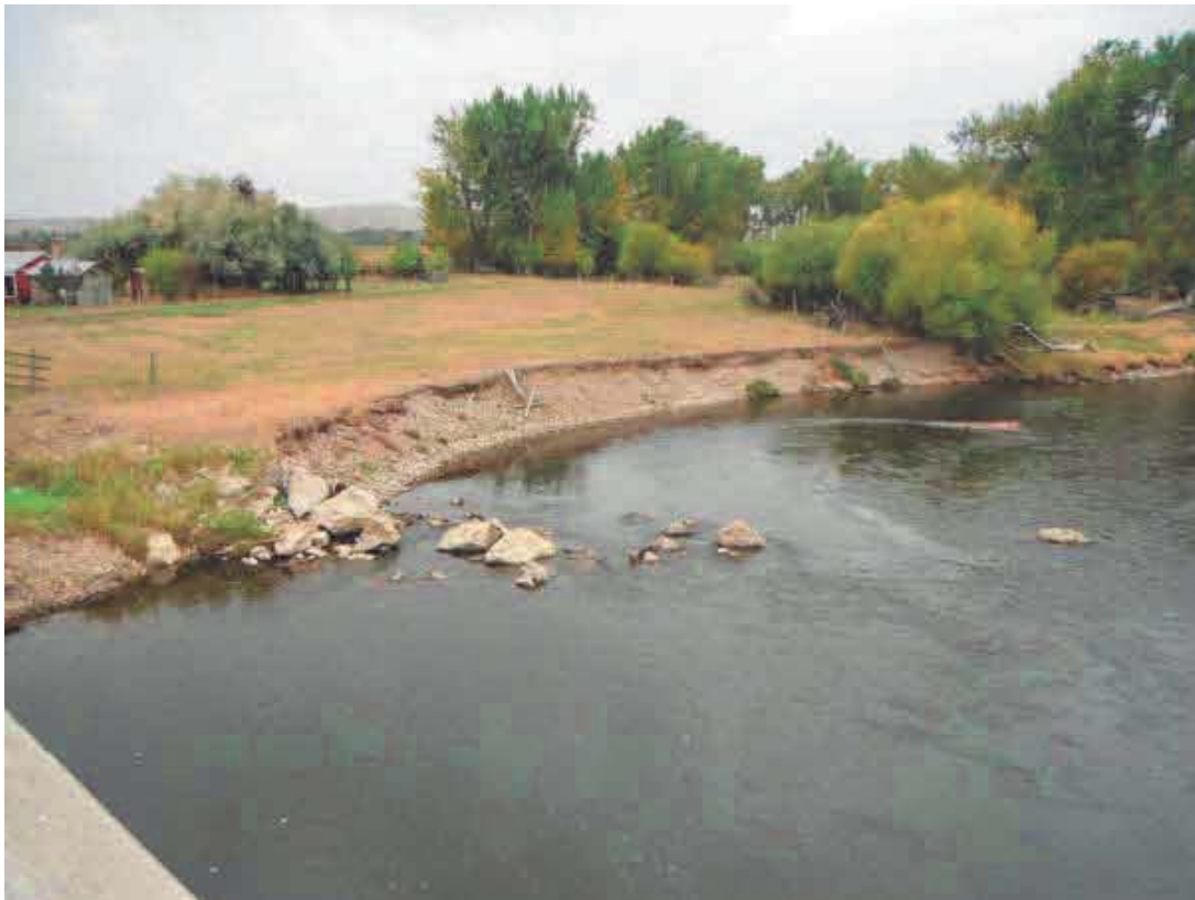
Figure 3. Right bank of Sub-Reach 5 in September 2015, prior to bank stabilization (riprap) placement. View from upstream rail of Pennington Bridge.
